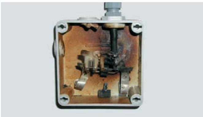
Module box after lightning strike
